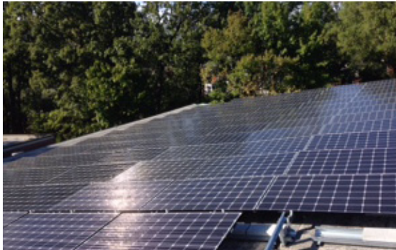
Solar panels installed on racks on the temple roof
