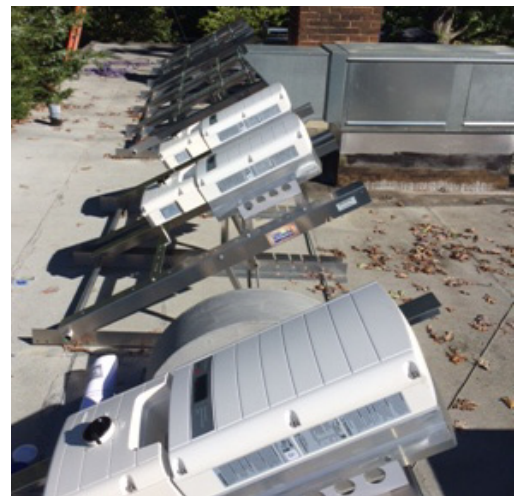
Inverters on the temple roof that connects our solar power with the PEPCO energy grid.
